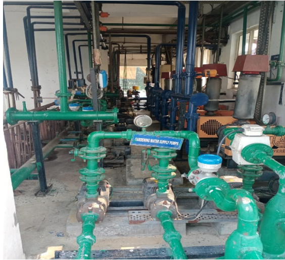
Figure 4 Gardening water supply pumps for reuse of treated water
