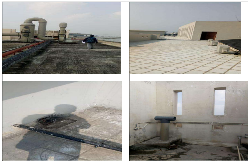
Figure 7 Rooftop rainwater harvesting
