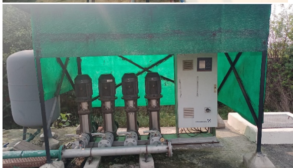
• Figure 3 Shiv Nadar University Sewage Treatment Plant
