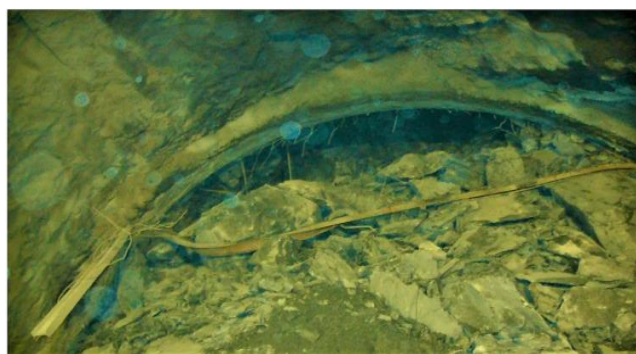
Picture 2 Landslide inside Bayu Tunnel
