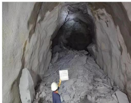
Picture 1 Rock Burst in Bayu Tunnel
