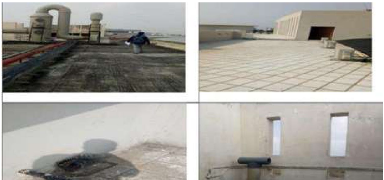
Rooftop Rainwater harvesting
