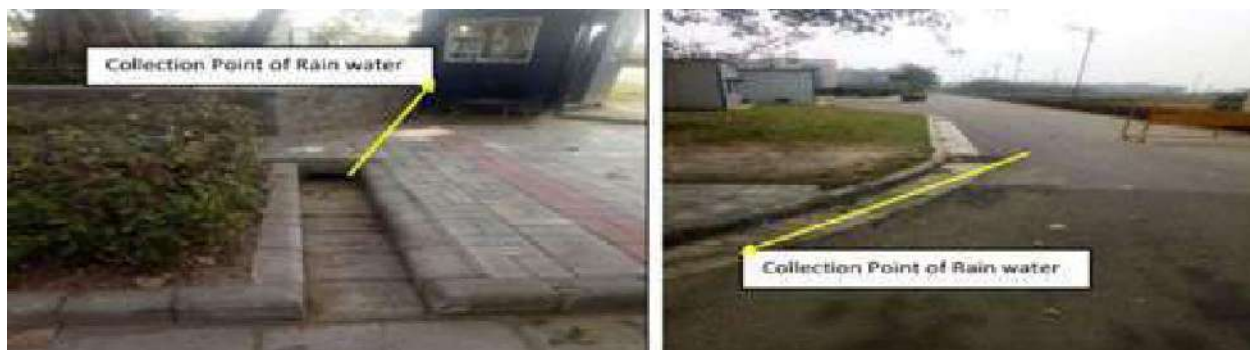
Stormwater drainage and catchment
