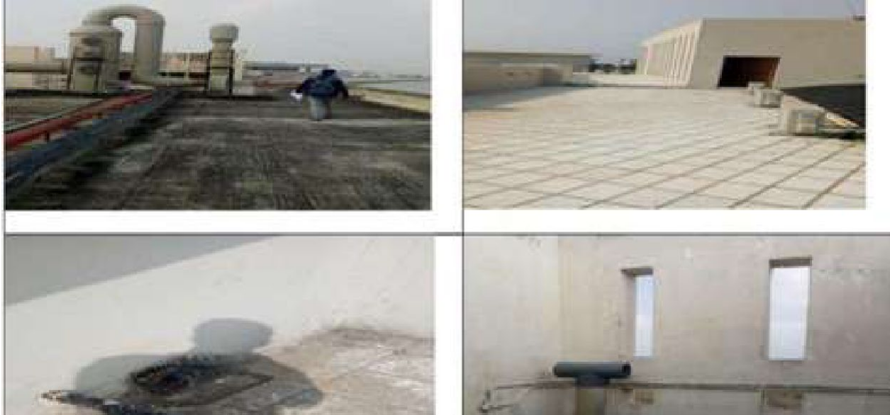
Rooftop Rainwater harvesting
