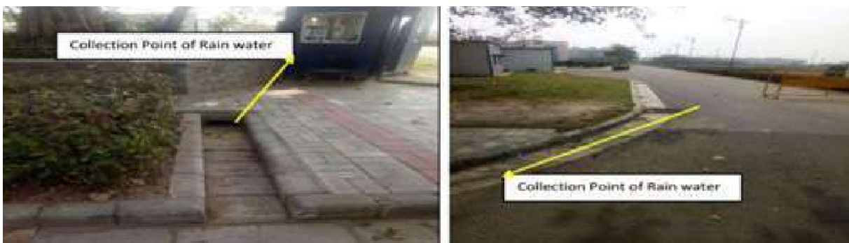
Stormwater drainage and catchment
