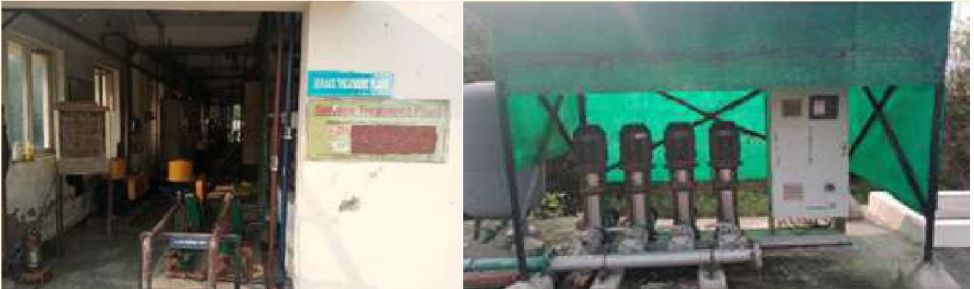
Sewage Treatment Plant on campus
