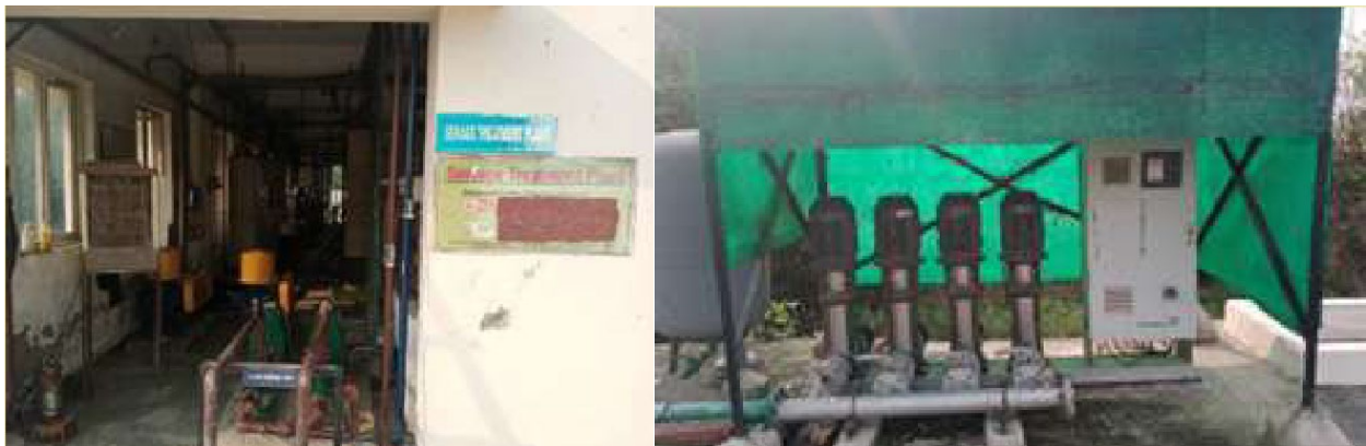
Sewage Treatment Plant on campus
