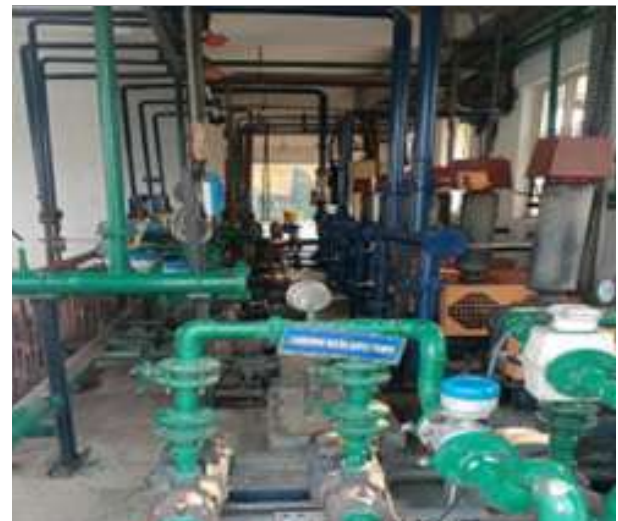
Gardening water supply pumps for reuse of treated water
