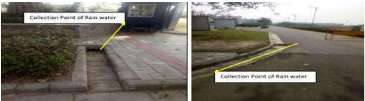
Stormwater drainage and catchment
