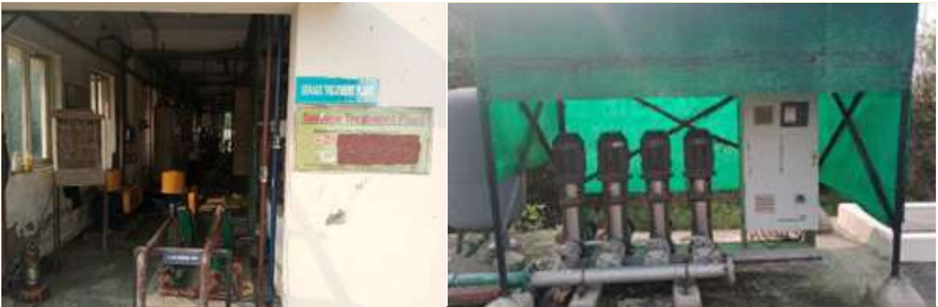
Sewage Treatment Plant on campus
