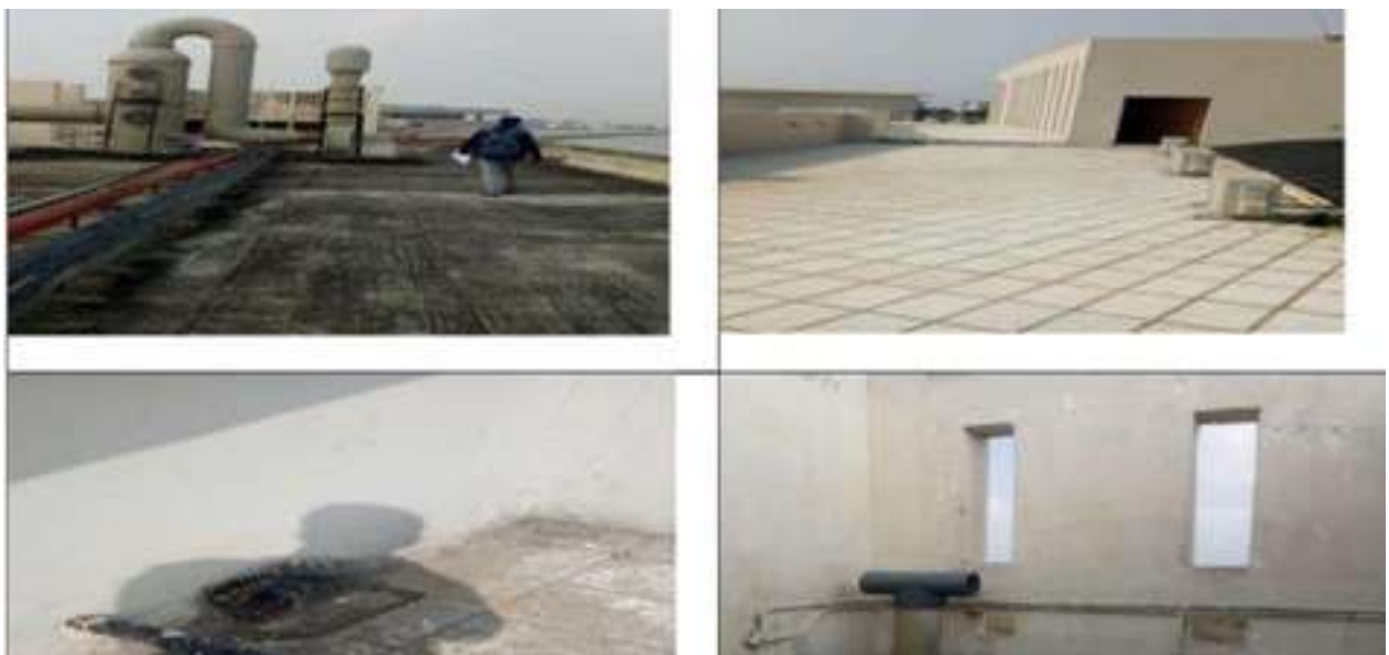
Rooftop Rainwater harvesting
