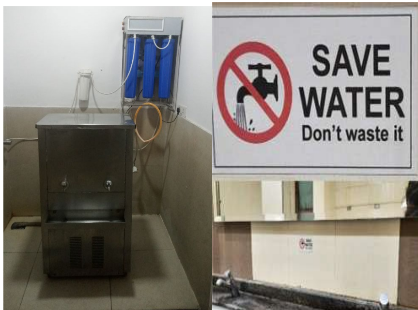
Water dispensing units are fitted with filters and display signage
